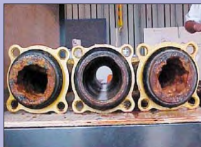
Biofilms in water pipes can harbour disease-causing bacteria and increase corrosion
